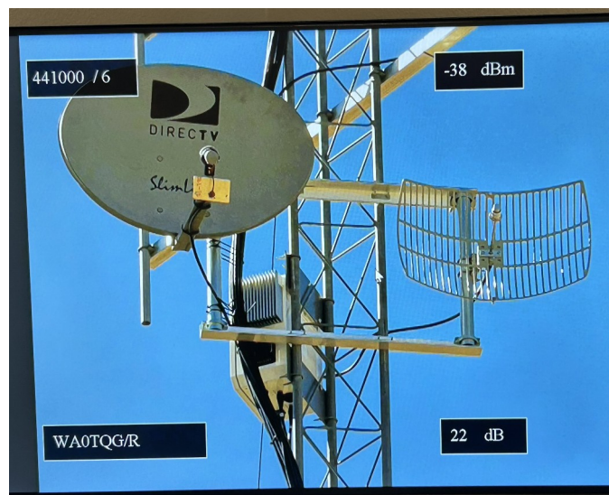
10 & 5 GHz dish antennas plus tower mounted electronics package
